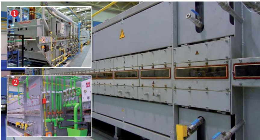
Roller hearth furnace for sintering process up to 2336 °F
